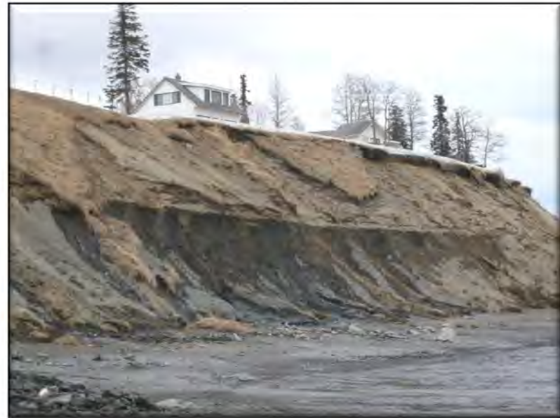
Bluff Erosion along Kenai River
