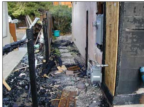
Figure 1. The gate that was attached to the garage at the corner ignited and led the fire to the home, causing the damage seen here ( firecenter.berkeley.edu ).
