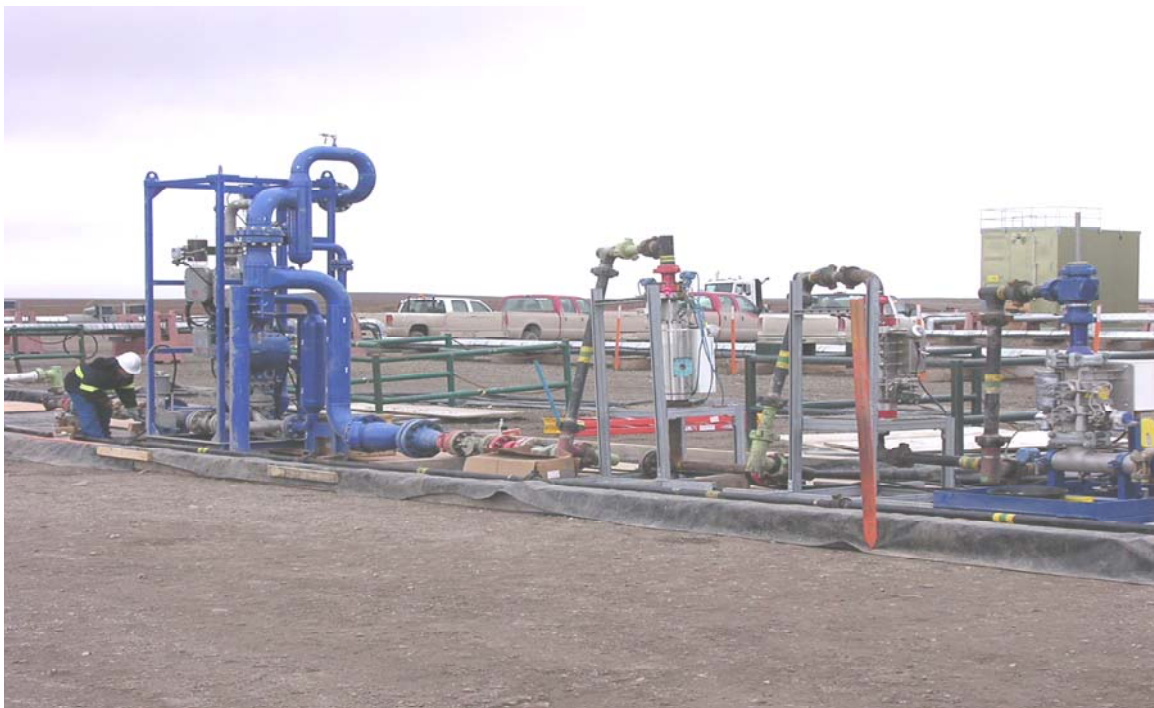
Figure 5 – A field test loop that includes four different multiphase metering systems. From left to right- Agar MPFM 400, Roxar 1900VI, FMC FlowSys, and Schlumberger Venturi X. (21)
