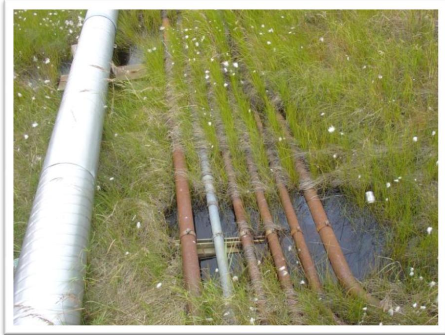
Photo 23: Fuel piping along ground in central part of community
