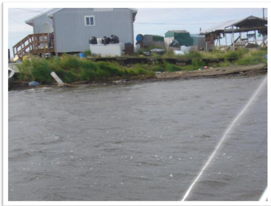
Photo 20: Riverbank erosion near existing structures and undermining boardwalk.
