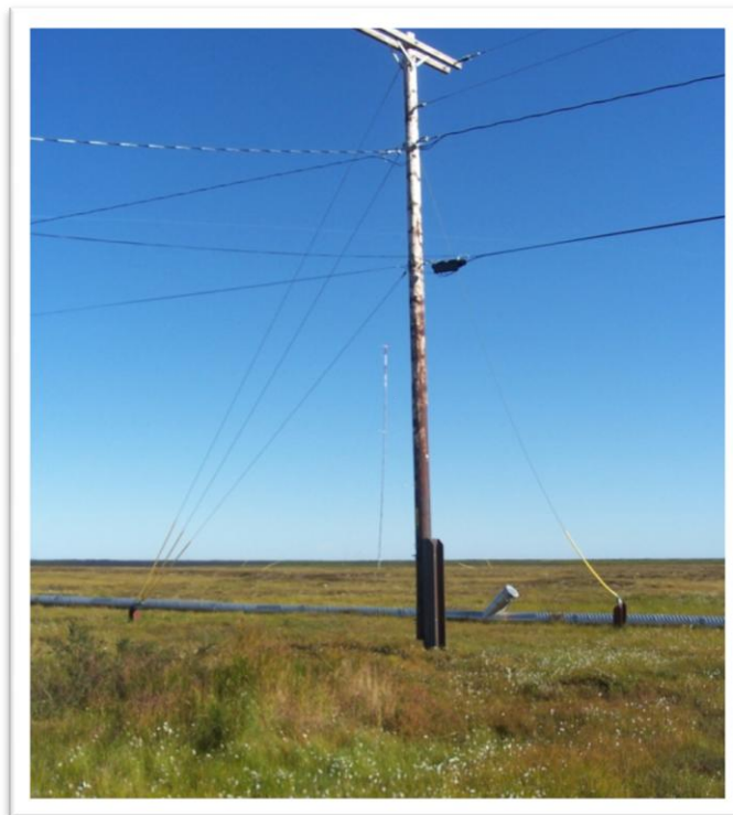
Photo 26: Utility pole on H-piling support with slack guy wires
