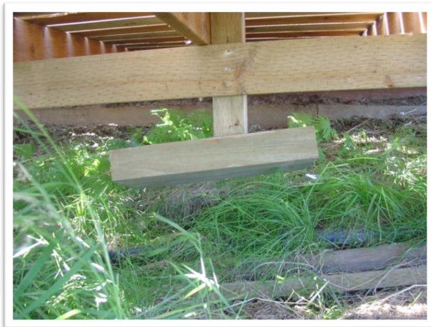
Photo 8: Floating footing under lift station. Given the lack of discoloration that would be an indicator of embedment, the pad may have been supported on blocks in the past, rather than being an indication of settlement.
