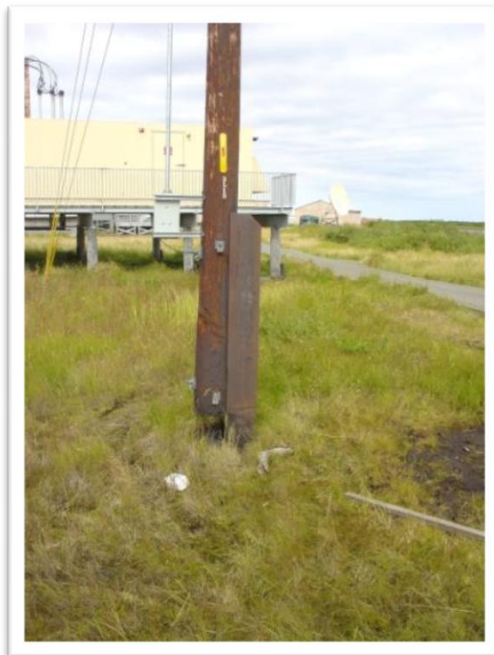
Photo 4: Timber utility posts have been cut off near the ground surface and attached to H-piles. We understand this work was completed within the last few years.
