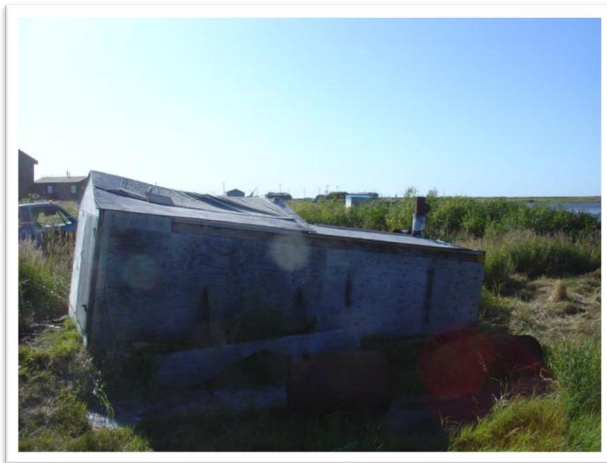
Photo 22: Smoke shed undergoing settlement near lake on north side of village.
