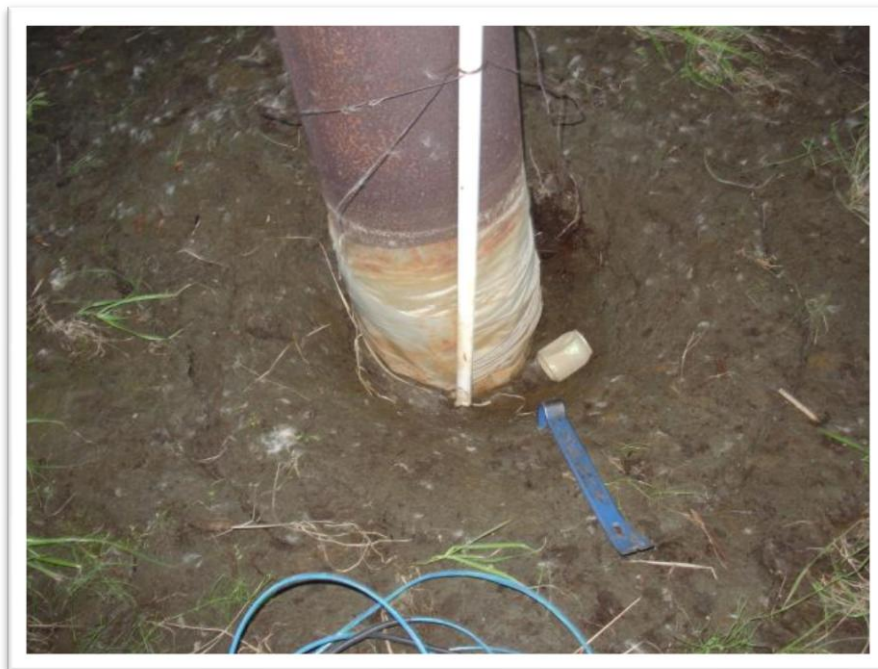
Photo 12: Settlement around wrapped steel pile under the fuel storage area.
