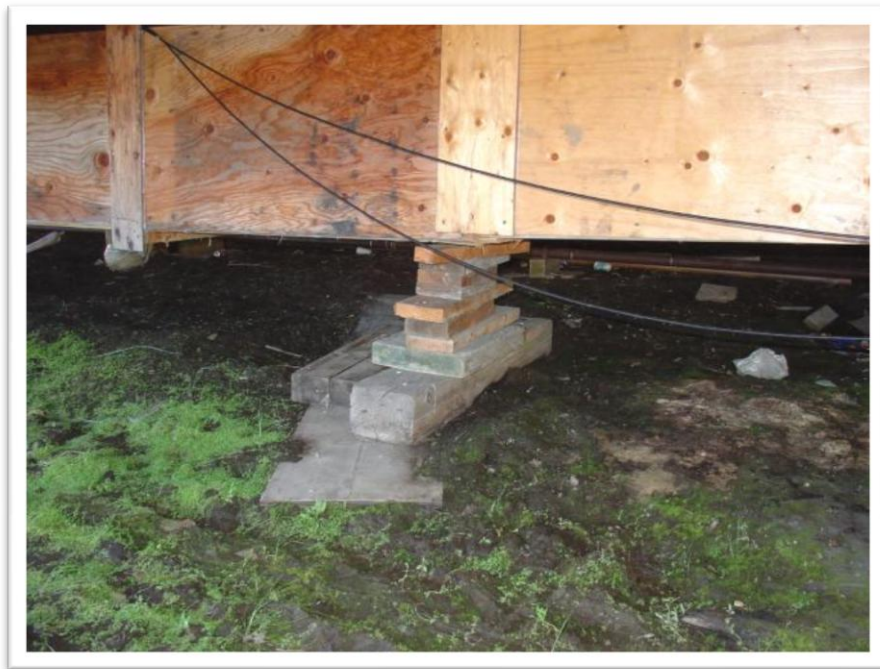
Photo 6: Blocking under school.
