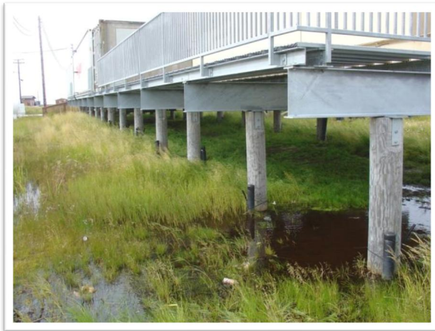
Photo 2: Timber piles supporting generator and electrical support pad. Note ponded water near piles. We attempted to measure temperature in black PVC pipe, but the water in the casing was frozen at a depth of approximately 2 feet.
