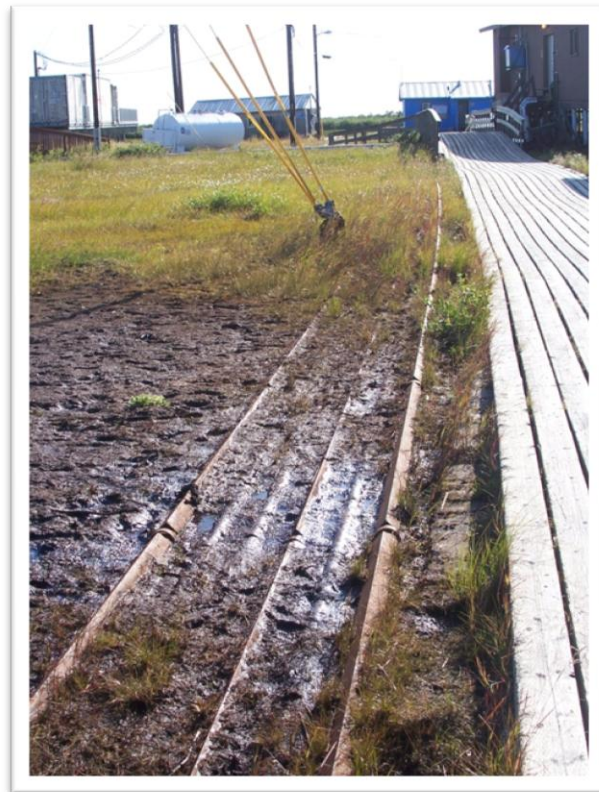
Photo 24: Fuel piping along ground in central Atmautluak
