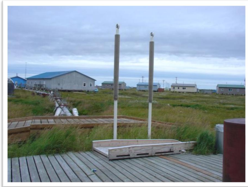
Photo 5: Passively refrigerated thermosyphons near the sewage lift station, sewer line in background.
