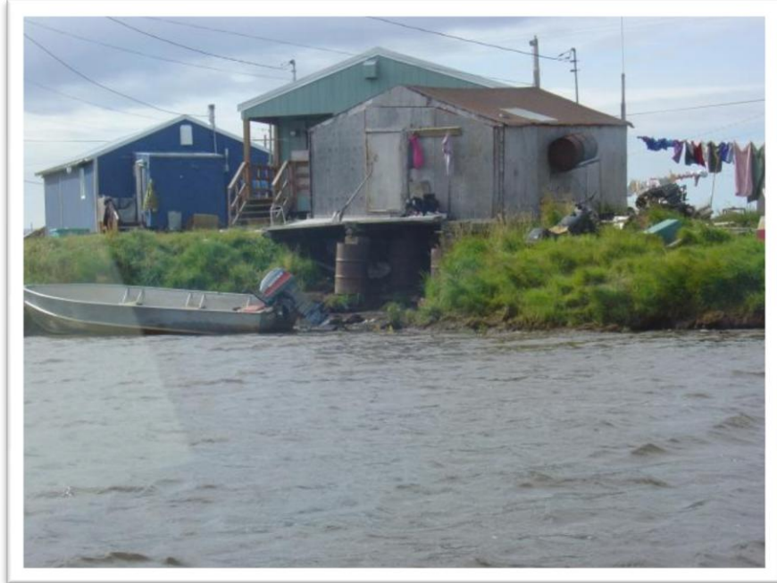
Photo 19: Riverbank erosion under existing structure. Building is being supported, in part, on fifty-five gallon drums.
