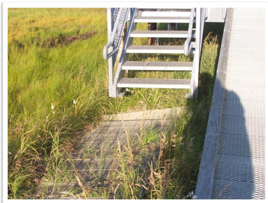
Photo 30: Stairs at National Guard Armory no longer reach ground level.
