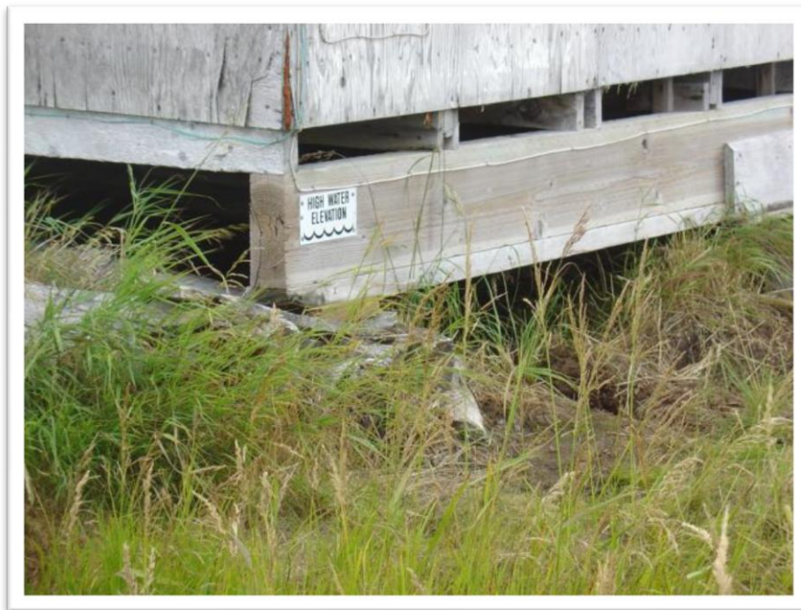
Photo 18: Close up of high water elevation mark on residence. Note apparent timber (non-pile) foundation.
