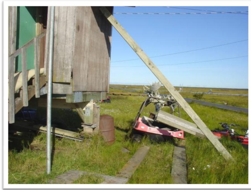
Photo 9: Repair of distressed residence near north end of village. Note blocking between pile top and support. The diagonal member appears to provide lateral support to the entryway.
