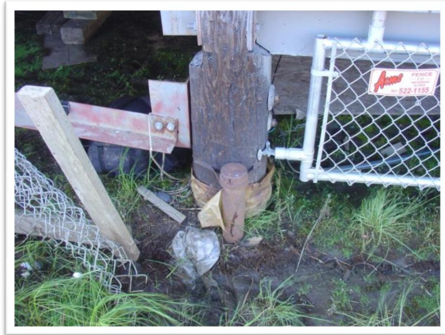
Photo 7: Plastic-wrapped wood pile supporting the school building. We attempted to access the pipes alongside the piles to measure temperature, but either could not remove the caps or they were blocked by ice at about two feet below the surface.
