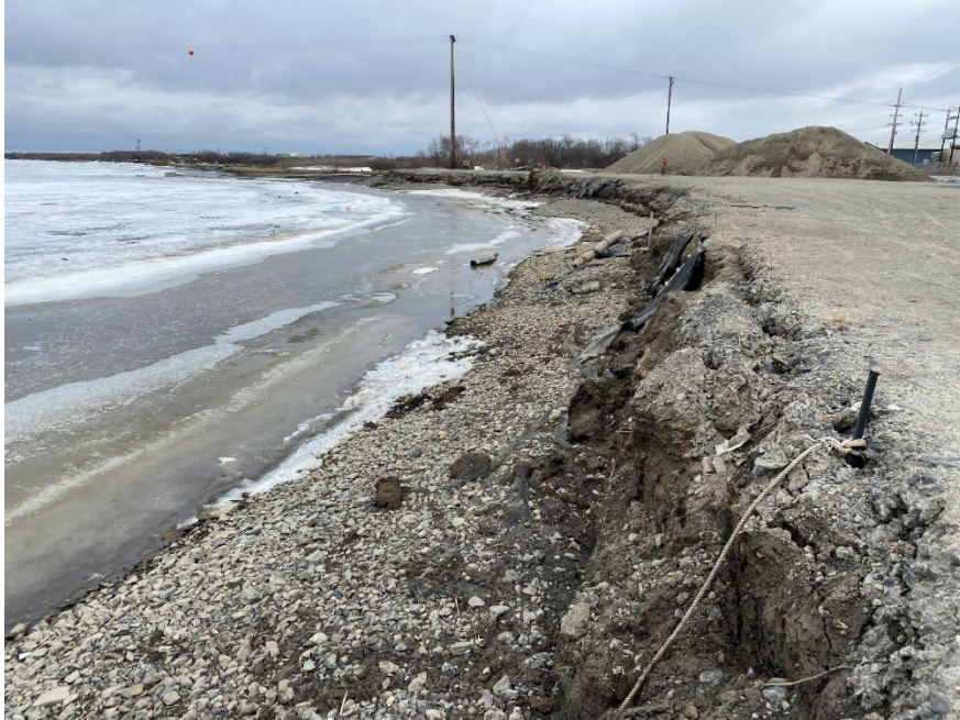
Figure 4: The image above shows the eroding shoreline near the barge landing and the water intake. This is the area with the highest erosion rate.
