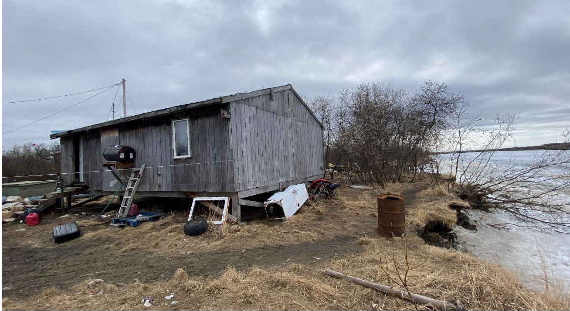
Figure 8: The home above is the most imminently threatened structure in Alakanuk and is approximately 12 feet away from the shoreline. Source: ANTHC.
