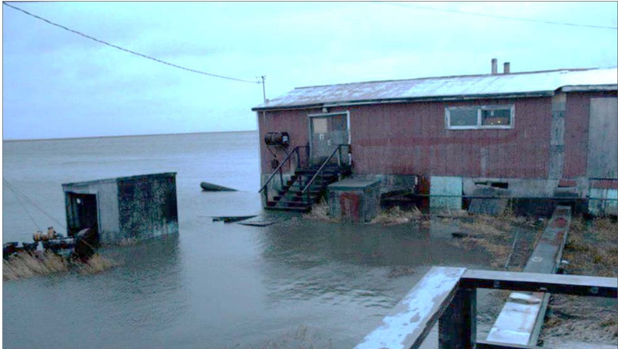
Figure 10. Flooding of Head Start Utility Building, morning of October 5, 2017
