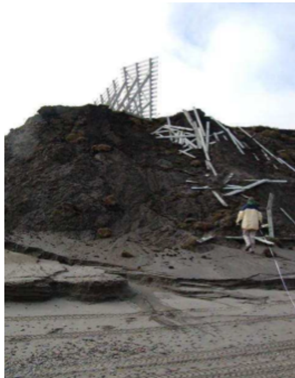
Figure 5: Shoreline Erosion (Source: Army Corps)
