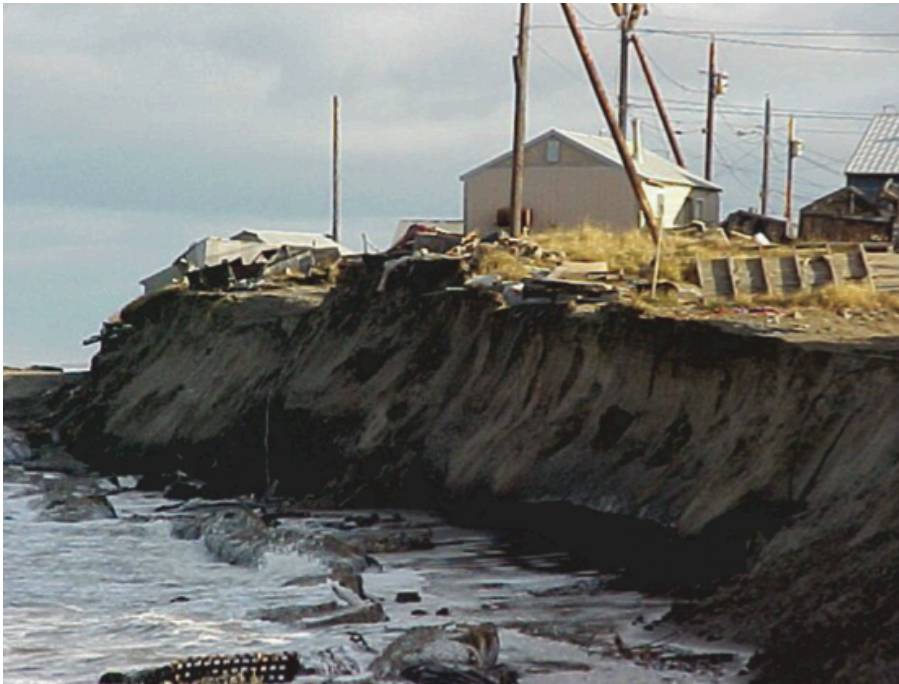
Figure 2: Bluff Erosion and Permafrost Melting in Shishmaref c. 2002 (Source: Kawerak)
