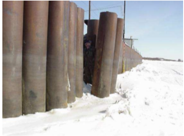
Figure 6: Pile wall of current concern at Bethel (Source: Army Corps)
