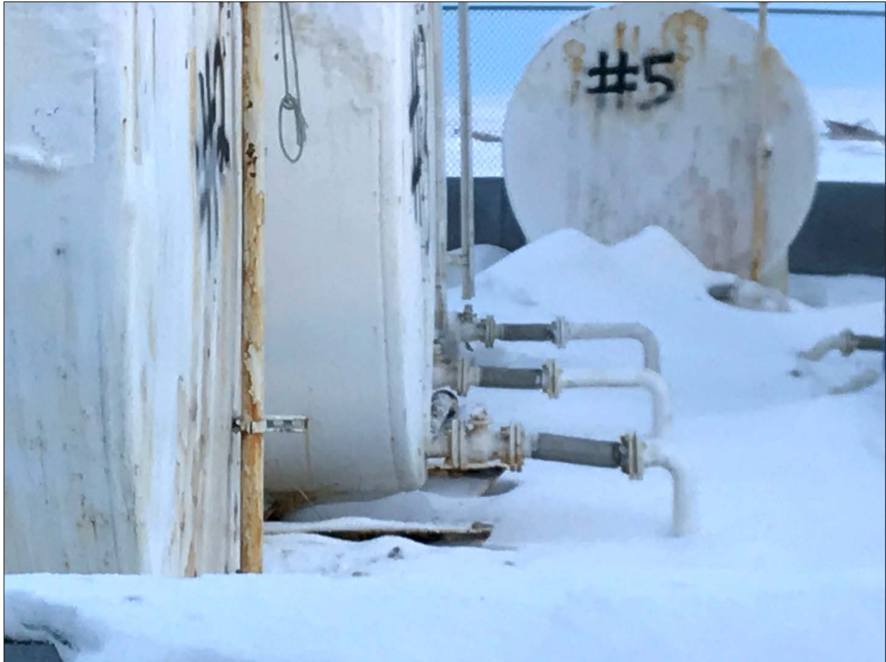
Figure 18. Settlement of Tanks
