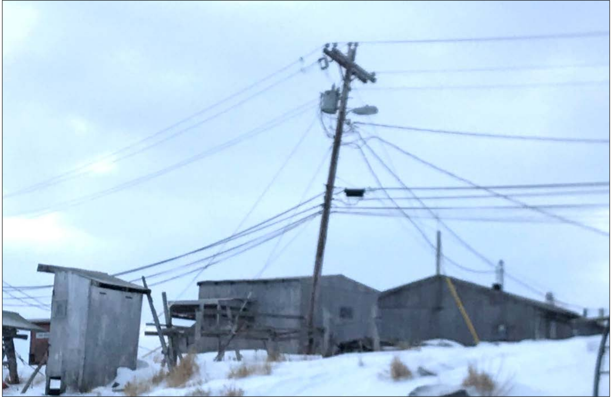
Figure 19. Heaved and Leaning Power Pole
