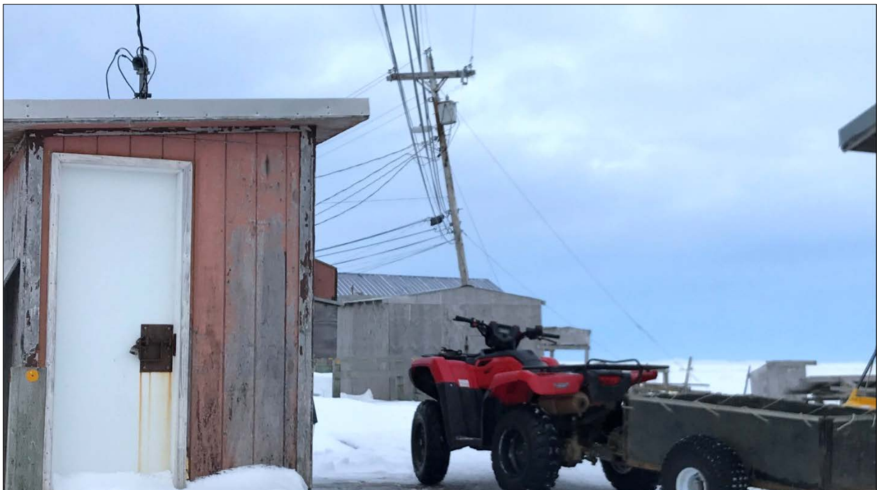
Figure 20. Heaved and Leaning Power Poles
