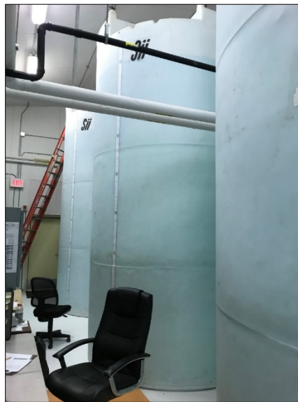
Figure 15. School Water Supply (Desalinated)
