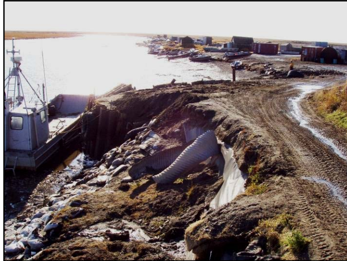
Figure 6.6.11: Erosion of the access road and sheetpile dock area at Chevok.
