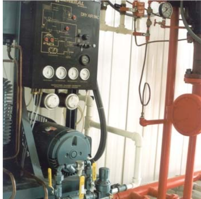
Compressor for Dry Pipe Sprinkler System
