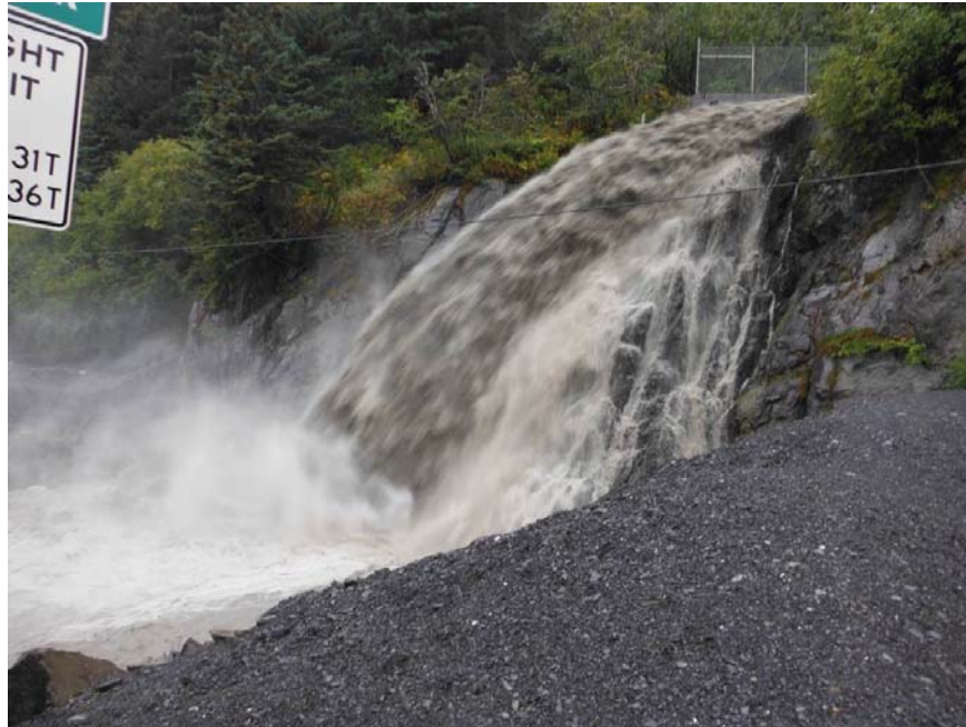
Figure 5-10 Lowell Creek Tunnel Debris Laden Outfall (URS 2012)
