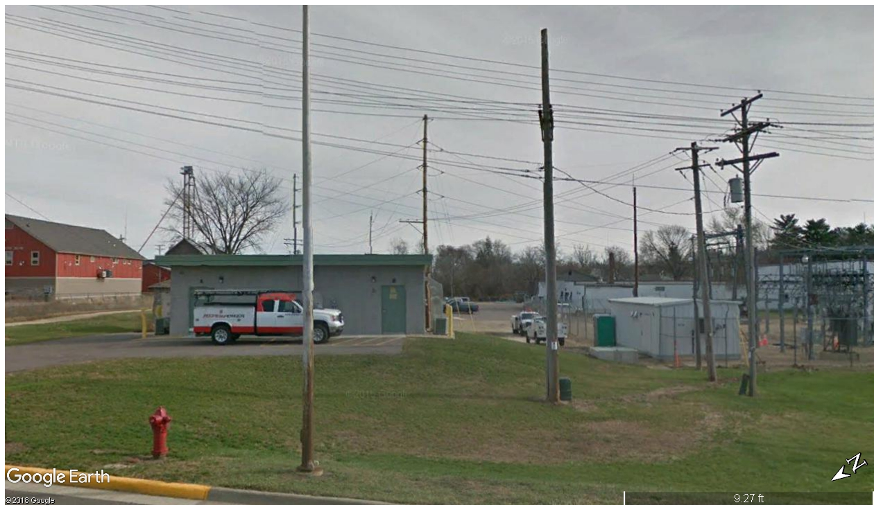
Figure 21. Electrical and telephone switching stations in Reedsburg, Wisconsin. The old one is to the right with the green cabinet next to it; the new one is to the left, behind the pickup truck.
