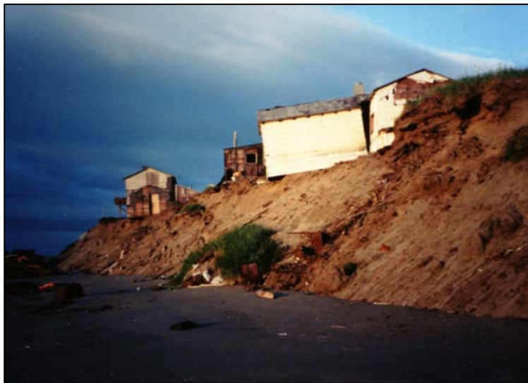
Erosion in 2000, has been an ongoing problem.
